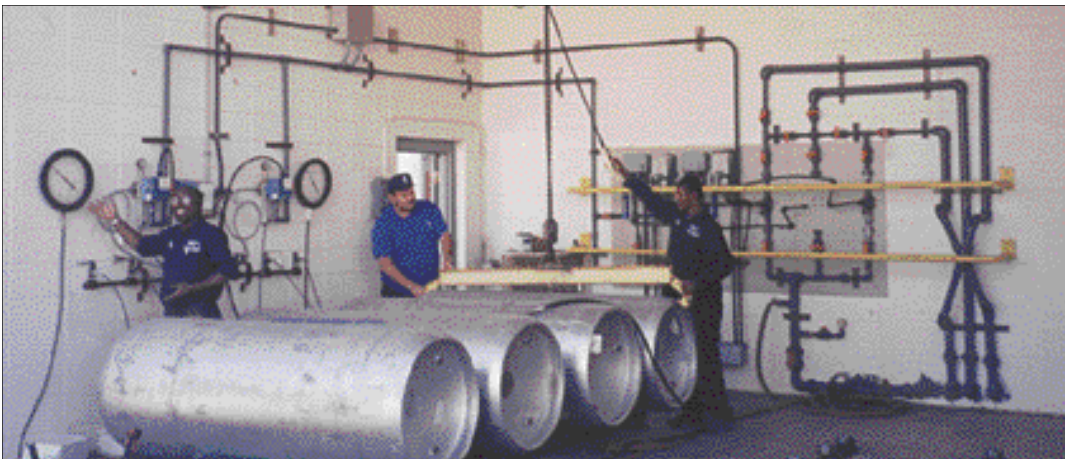
Employees at the Freshwater Treatment Plant check the chlorine tanks vital to the process of providing residents with safe drinking water.
