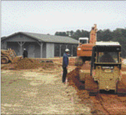
Some landscaping work will add grass, shrubs and flowers to complement the new pavilion at Bonita Lakes.
